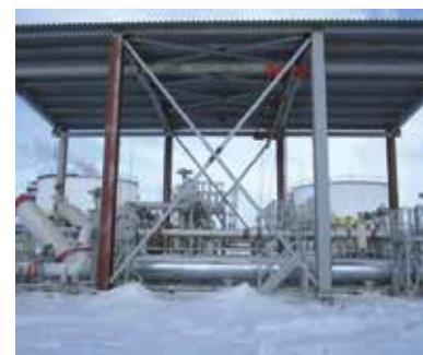
Metering system for Transneft Russia
