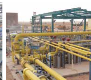
GRS station Hassi II Algeria
