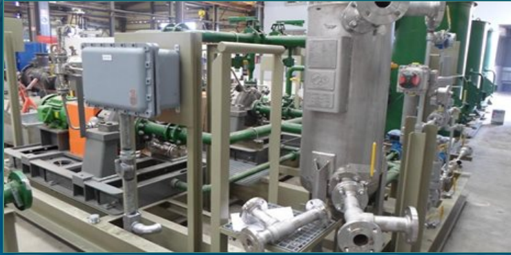
Pumps skids 102, 103 A/B/C and 104 A/B/C Carbutica district
