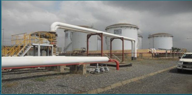
The new petroleum products storage and distribution terminal in Tema, Ghana
