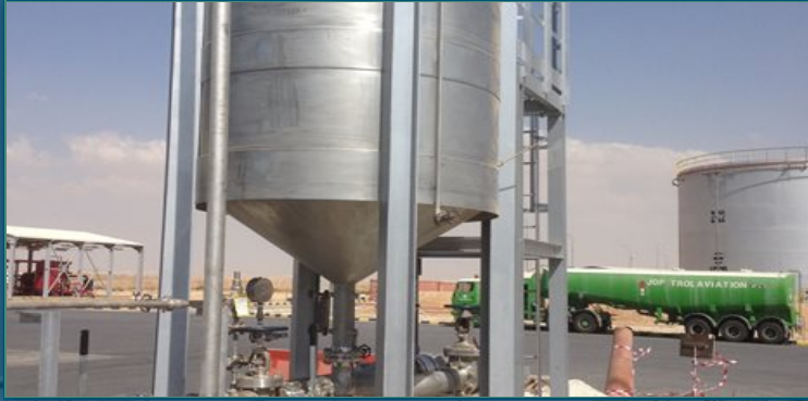
Test rig with prover tank Queen Alia international airport
